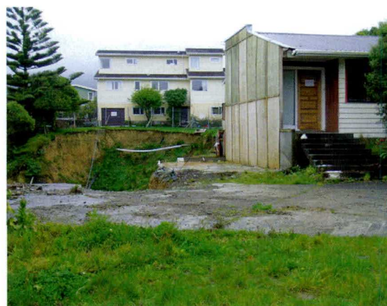
A large slope failure in Vista Grove, Kelson, Lower Hutt on 8 August 2006 generated nationwide media coverage. Four houses still remain threatened by the slip.
