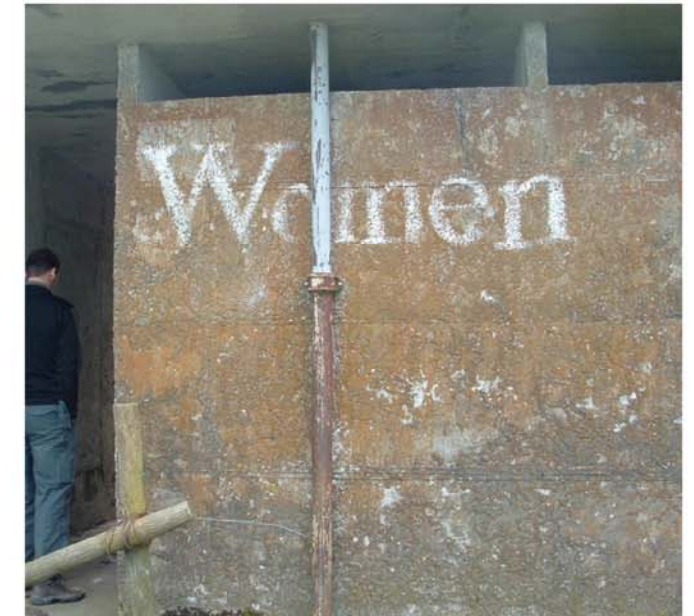
Lake Domain toilets are in a derelict state and require removal
