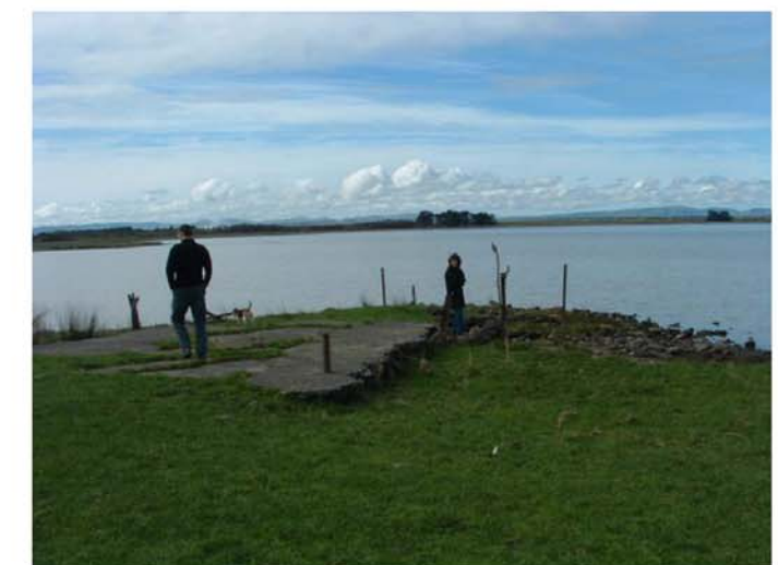
Boat launching ramp in disrepair
